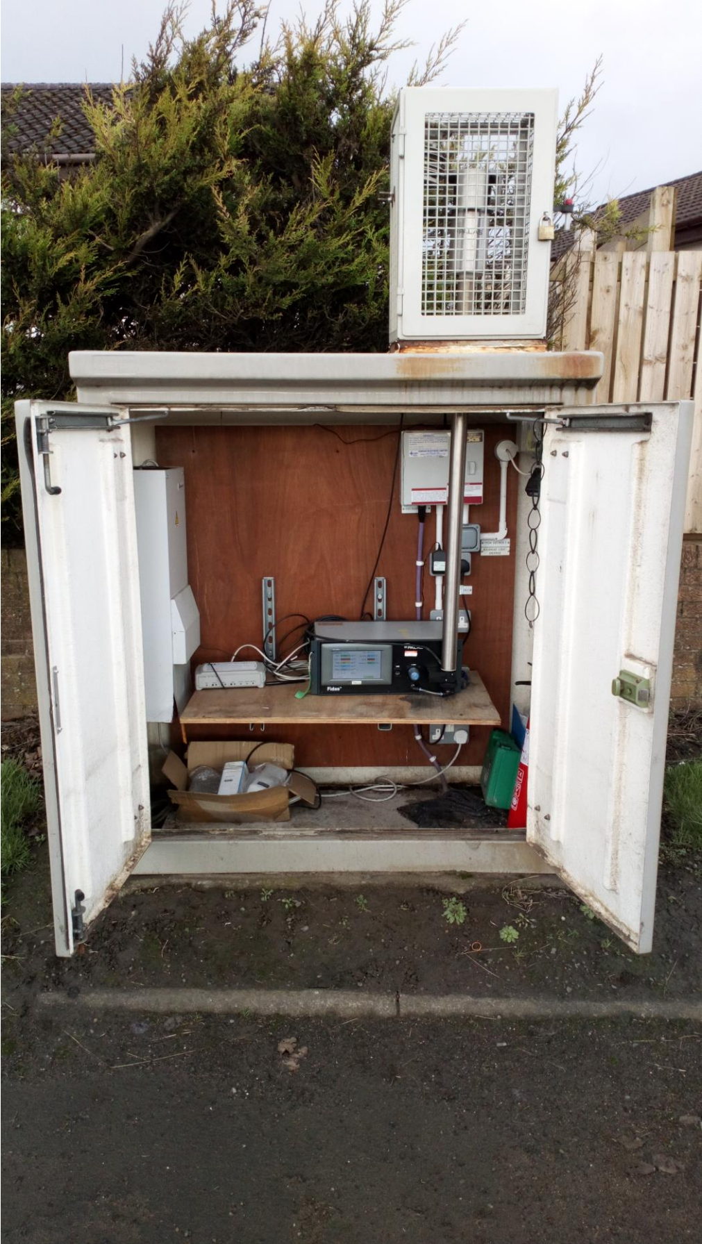
Photo 2 – Banknock 2 Automatic Roadside Station
