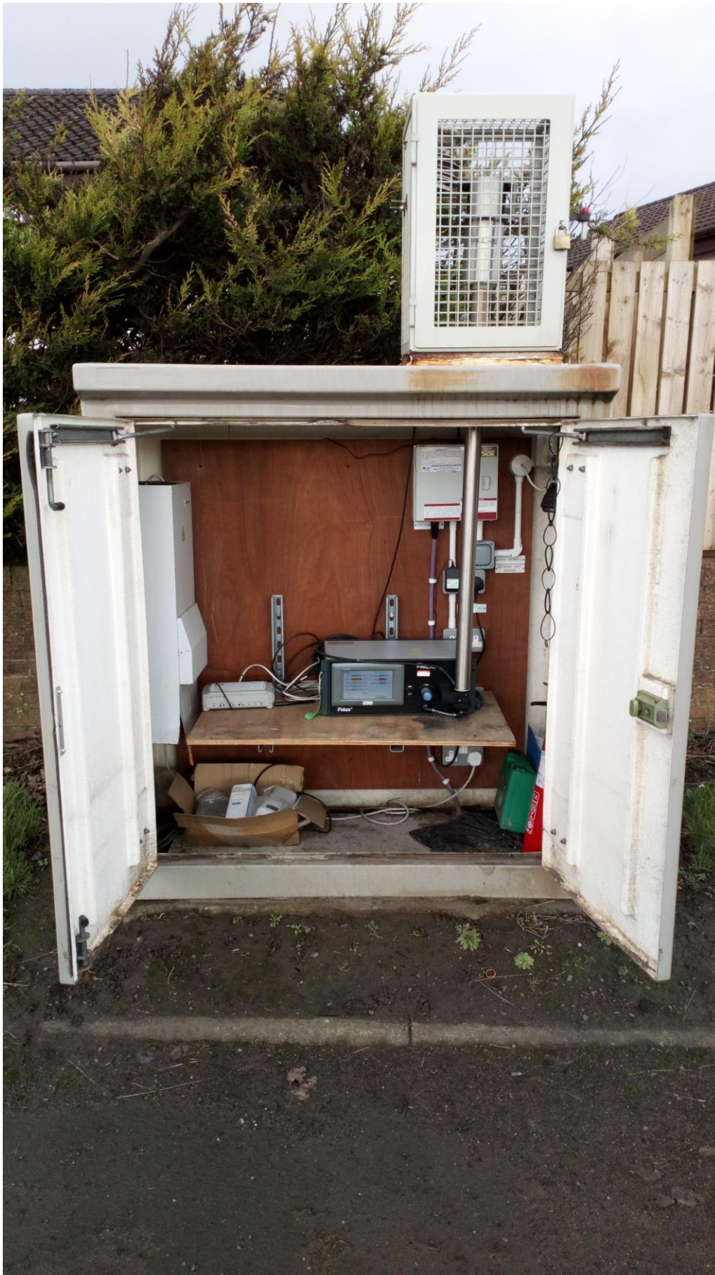
Photo 2 – Banknock 2 Automatic Roadside Station
