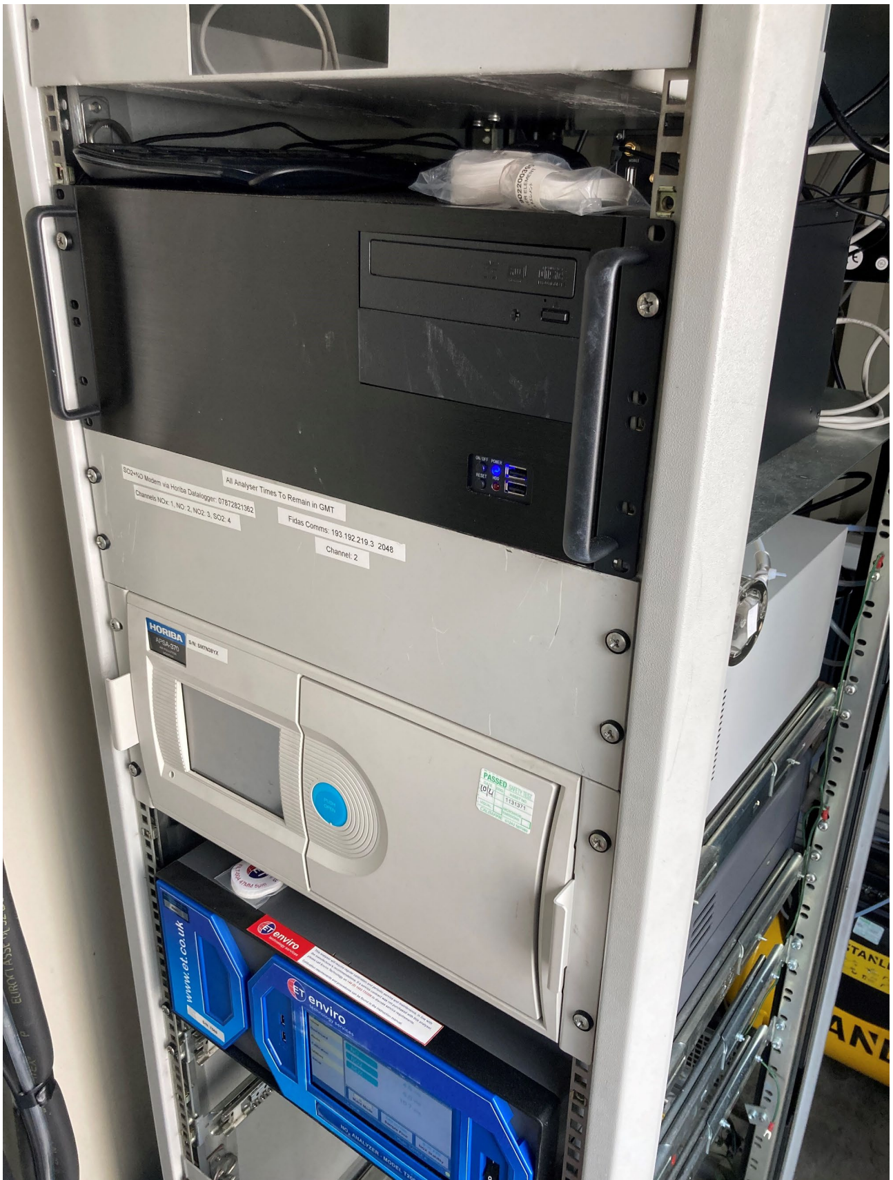
Photo 3: Rack Mounted High-Capacity Datalogger at Grangemouth Municipal Chambers Air Quality Station
