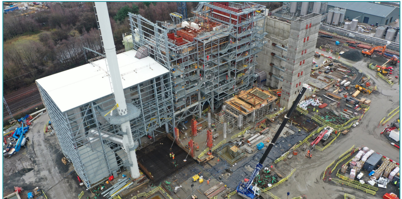
Copyright: Earls Gate Energy Centre
